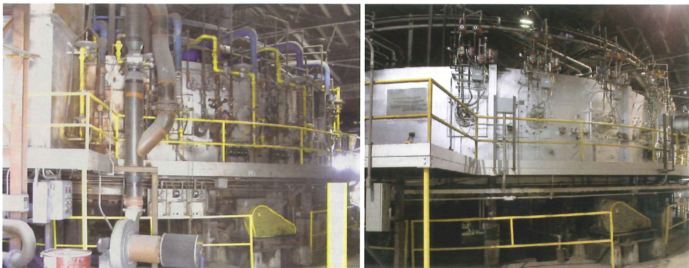
Fig. 5: Outside view of the rotary hearth furnace at ArcelorMittal Shelby, before and after the REBOX installation. Please note that all bulky equipment and piping relating to the previously used air-fuel system have been removed as it no longer is of any use
