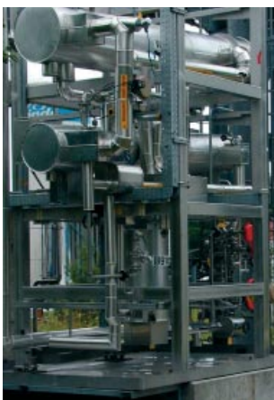
View of a cryo condensation plant
